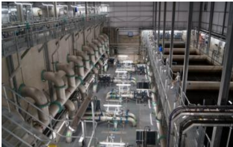
Picture 1: Dee Valley Water's £17m flagship water treatment works at Llwyn Onn, North Wales, is controlled from inlet-to-outlet by a Mitsubishi Electric system redundant, Q series modular PLC solution.
